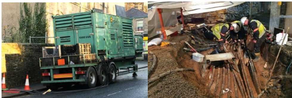
Figure 3-24: Response required due to substation flooding 23
